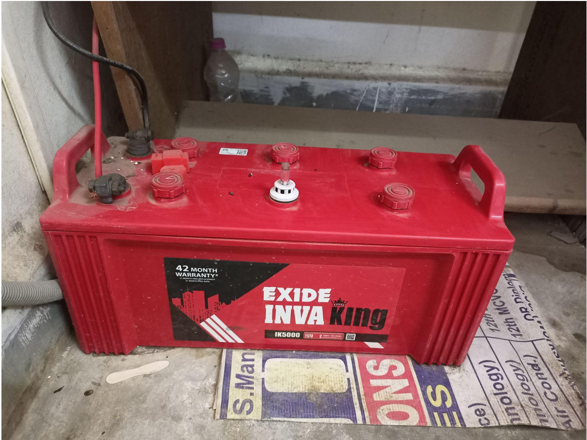
Exide Inva King IK5000 Battery for UPS Inverter to power College Server PC and Office PC
